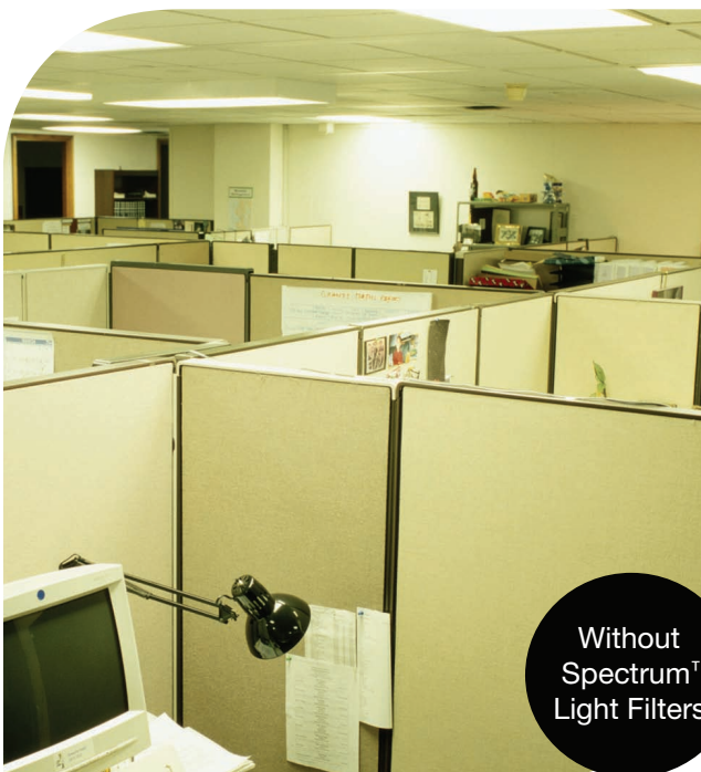
Typical office with fluorescent light installation
